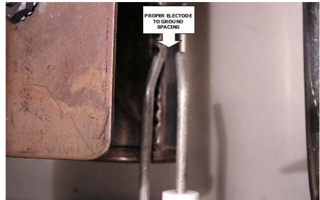
NOTE GAP ON ELECTRODE AND GROUND WIRE
